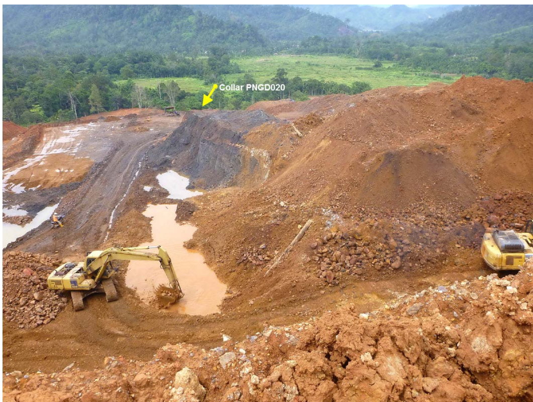
Figure 3: Location of drill hole collar for first drill hole at Kuini Prospect to test magnetite skin body (dark area) at depth. (Yellow arrow points to site and approximate orientation) View to northeast. Pit area is entirely with Prosperity ATP IUP.
